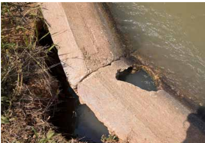
Damaged irrigation channel (M Mohell)
